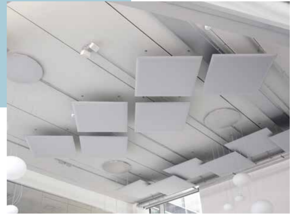
OVERSIZE / SNOWSOUND CEILING CABLES Caimi Lab Medtronic Italia, Milano (Italy)
